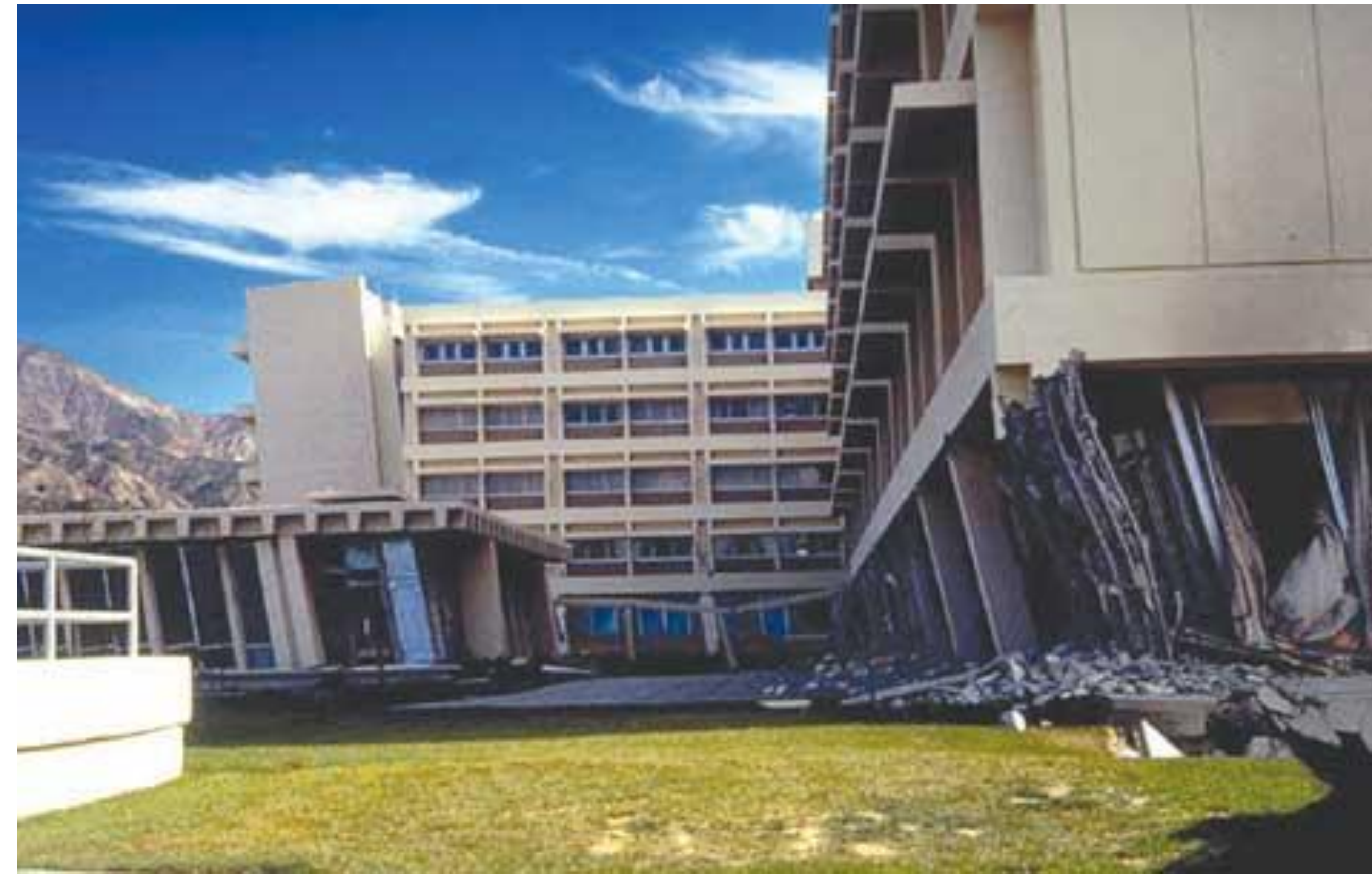
Olive View Hospital after the 1971 San Fernando Earthquake (Reference: CGS Website)
